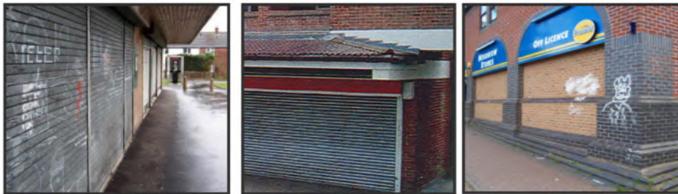
Poor quality shop fronts and steel shutters give a negative impression of an area and may be subject to graffiti.
