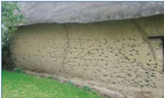
Earth walling is rare in the West Midlands but a small number of 'mud' walled farm buildings can be found in southern Warwickshire (Dunsmore and Feldon).
