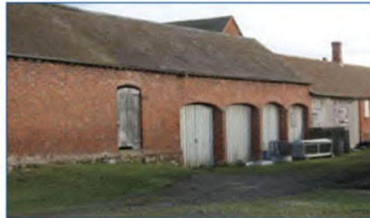
Cartshed bays set into the external wall of a regular planned farmstead (Shropshire, Cheshire and Staffordshire Plain).
