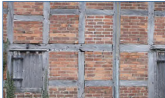
Timber-framing, here with brick infill panels, was a common method of constructing buildings until the 18th century (Herefordshire Lowlands)
