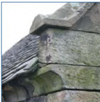
Detail of a fine eaves detail on the gable of a stone cow house (Potteries and Churnet Valley).
