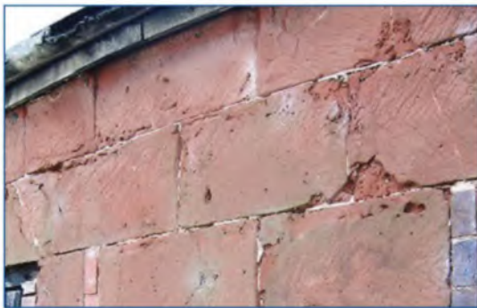
Old red sandstone used as ashlar is characteristic of north Shropshire and west Staffordshire (Shropshire, Cheshire and Staffordshire Plain).
