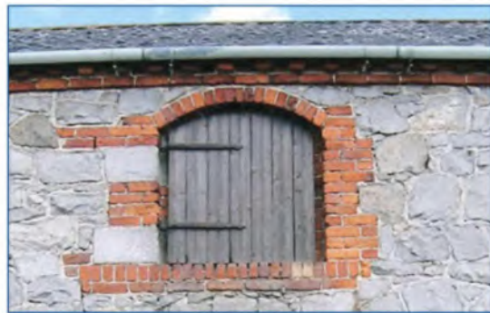
Stone rubble walling often has brick quoins and dressing to window and door openings (Shropshire, Cheshire and Staffordshire Plain).
