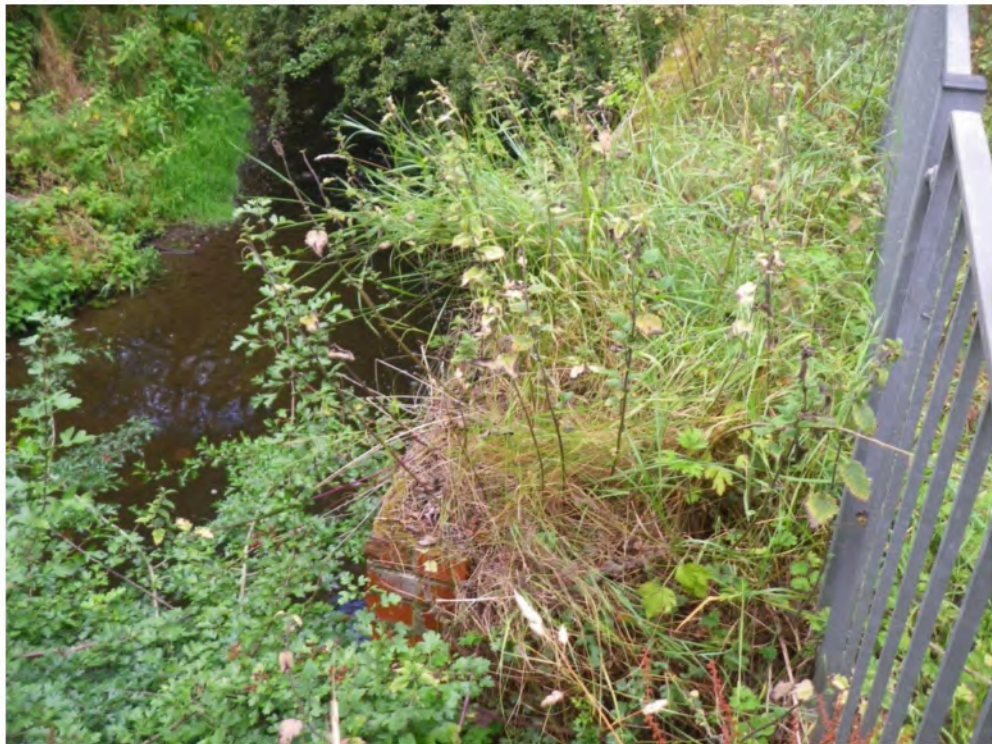
Photograph 14 - Flood defence at Paper Mill, Brooklands Lane, showing bank erosion
