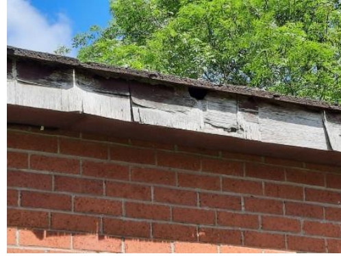
Plate 4.4: Hole in soffit
