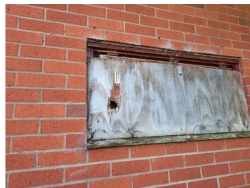
Plate 4.7: Boarded-up window with cavity
