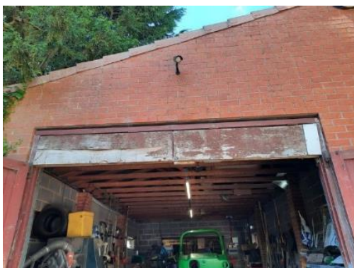
Plate 4.6: Gap above doors
