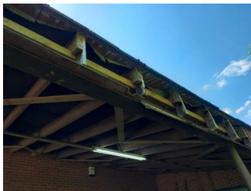
Plate 4.16: Damaged roof lining
