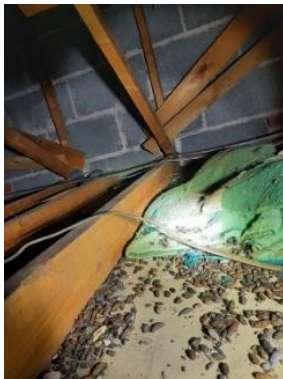
Plate 4.14: Rat droppings inside roof void
