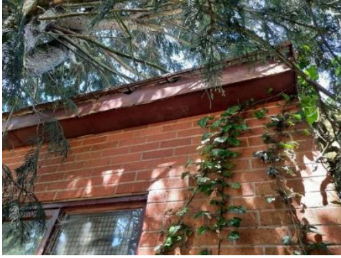
Plate 4.3: Holes in soffit
