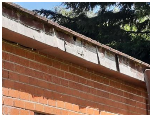
Plate 4.5: Peeling paint on soffit
