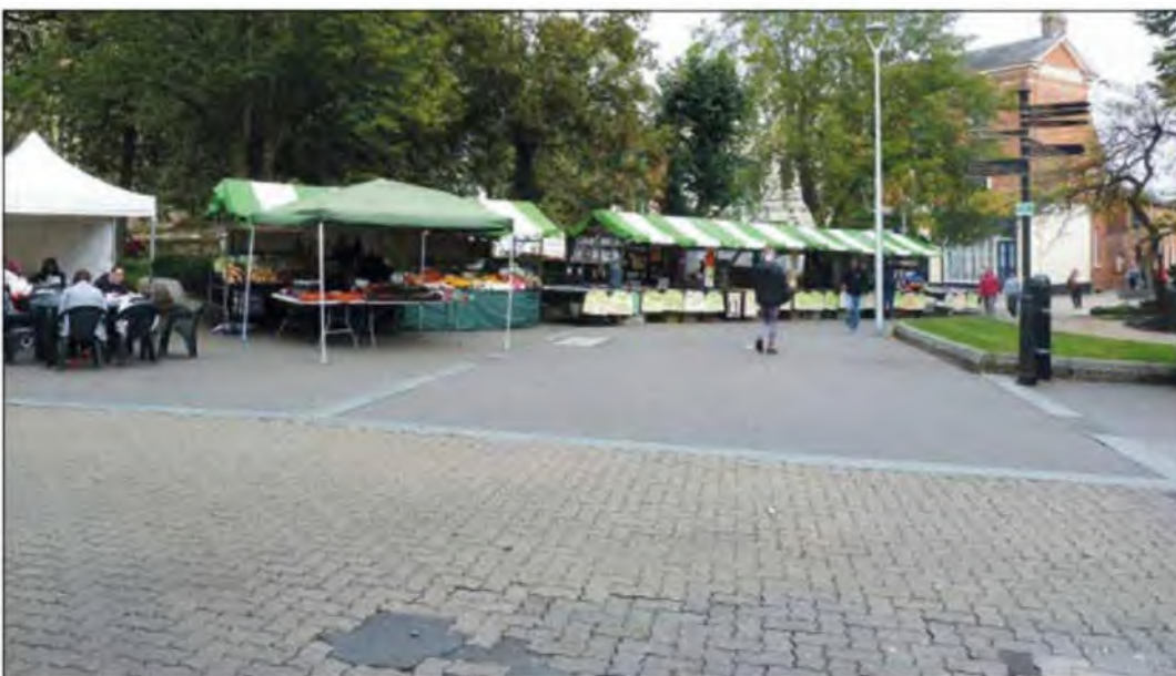
Patched block paving on Market Place
